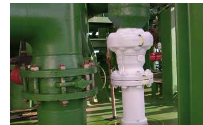
Transporte de amoníaco a baja temperatura Transport of ammonia at low temperature
