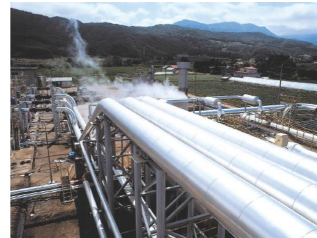
Geothermal steam pipe
