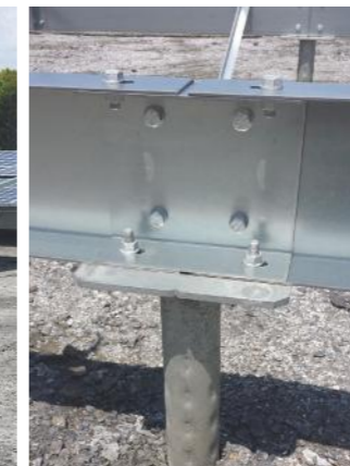
Dimple pipe for solar panel stand
