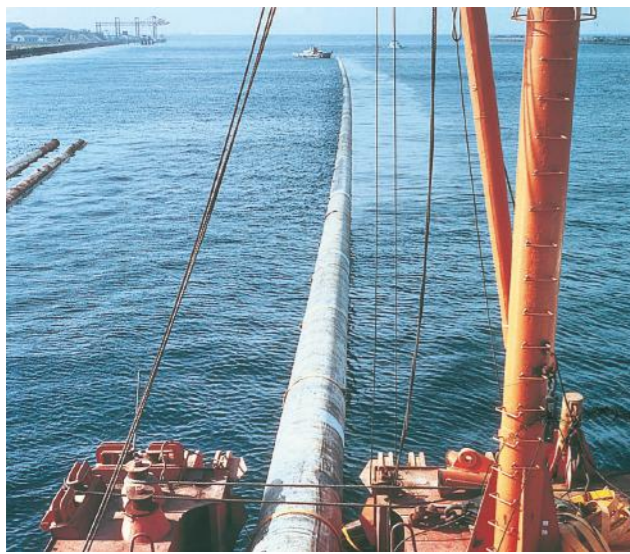
Offshore line pipes for receiving crude oil
