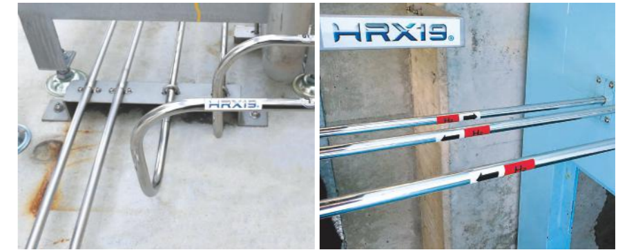
Hydrogen station piping
