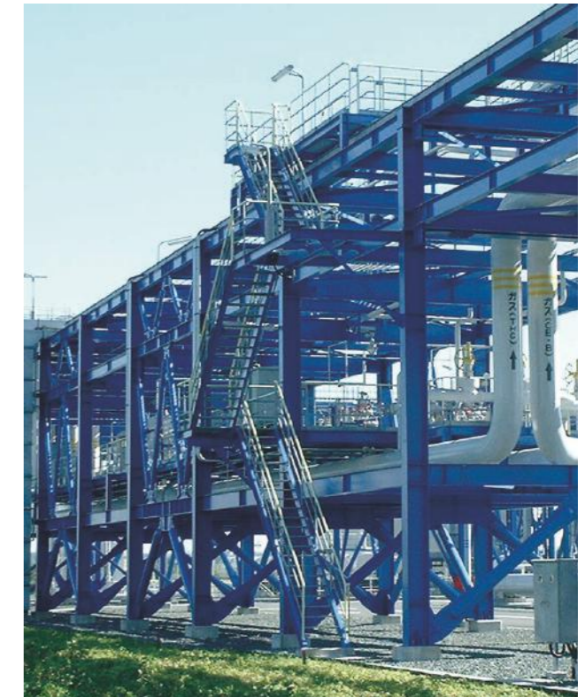
In-plant gas piping
