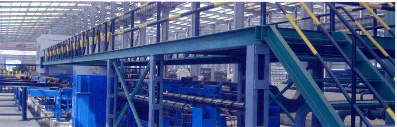
▶ 水压机3 Hydrostatic test machine
