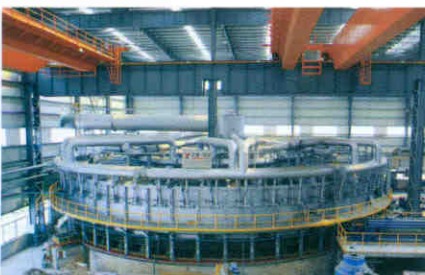
▶ 环形炉 Ring heating furnace
