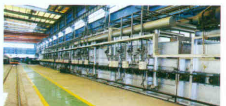
▶ \Phi 80 热处理炉 Heating furnace
