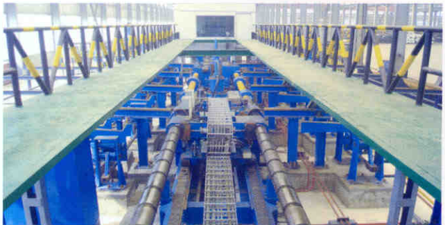
▶ 水压机2 Hydrostatic test machine
