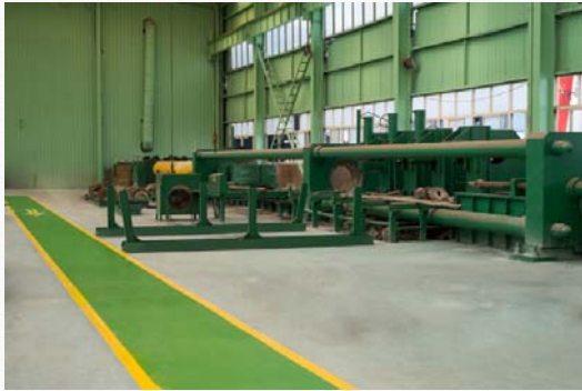
630mm Large diameter super-long hydraulic cold drawn stainless steel pipe production line
