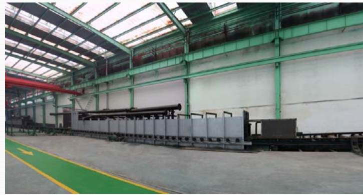
Four Automatic Natural Gas Annealing Furnace
